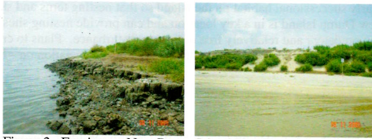
Figure 2. Erosion on New Dump Island (A – East side, B – West side).
