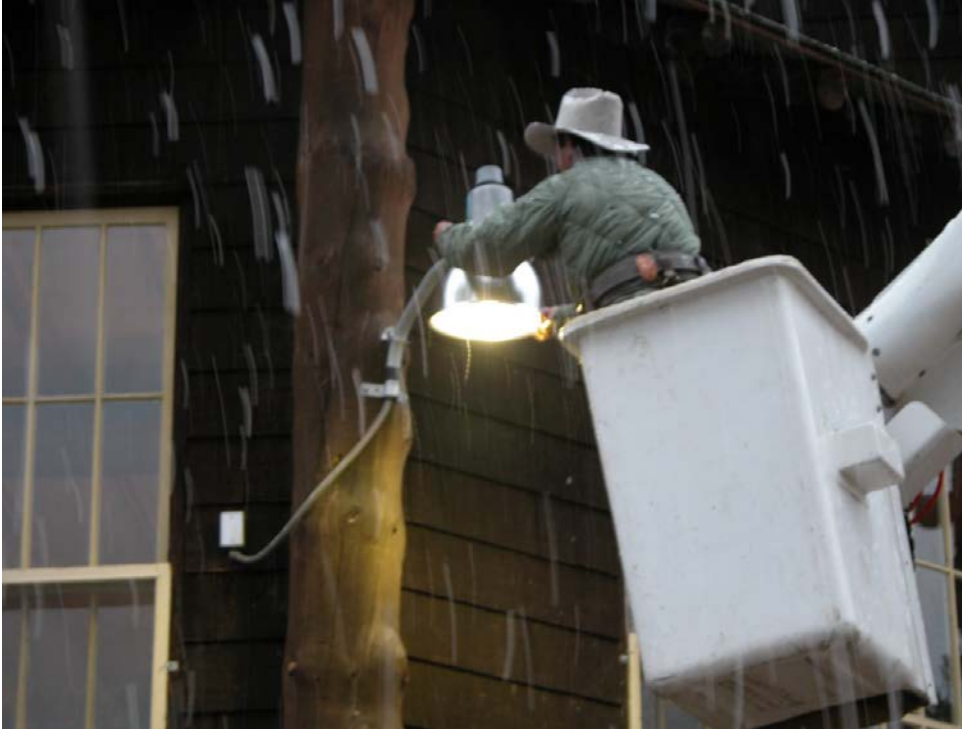
Figure 8. A full cut-off shield being installed on an existing light on the lodge at Yellowstone National Park. This previously unshielded light was visible across the lake and from the backcountry.
