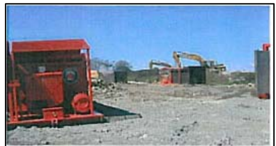
Air Curtain Furnace
